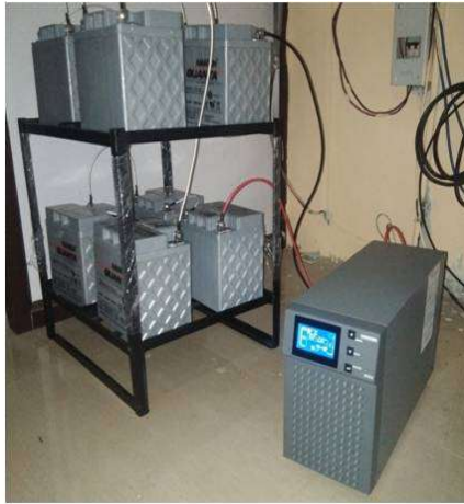
2Kva UPS Installed at Warehouse
