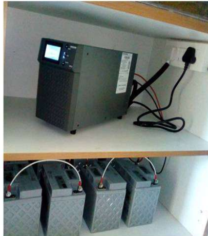
3Kva UPS Installed at Architect Office
