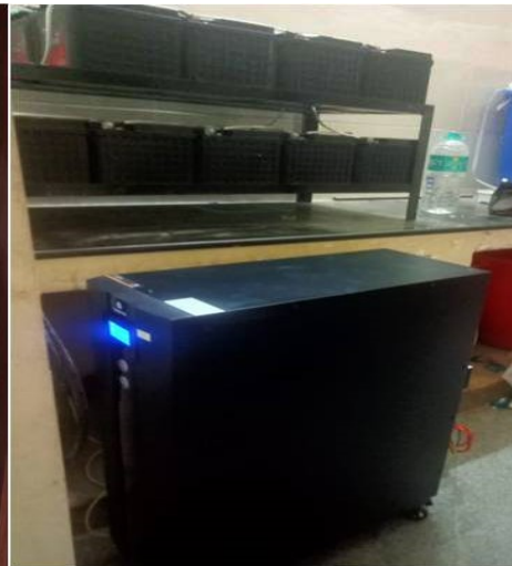
10Kva UPS Installed at Govt Hospital - Harapannahalli
