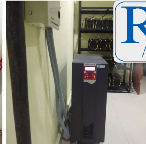
10Kva UPS Installed at SAI for Oxygen Monitoring System
