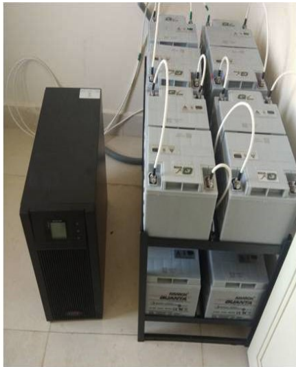
6Kva UPS Installed at Tumakuru Smart City
