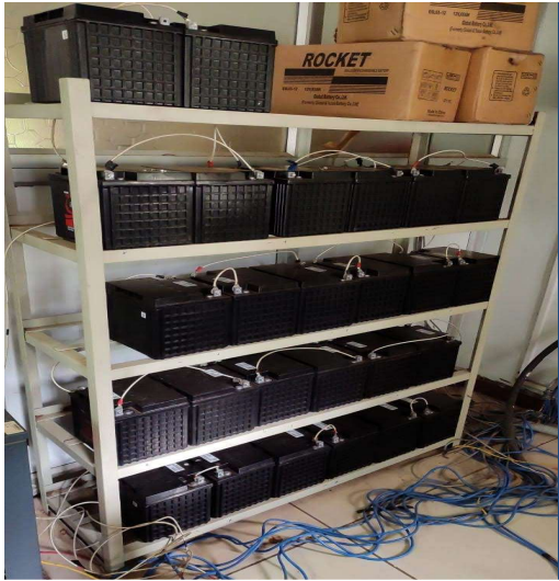
Installed Exide 42AH Battery - RTO
