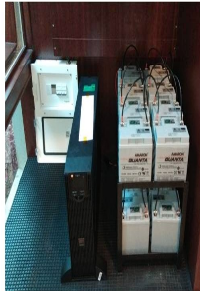
5Kva UPS Installed at Villa
