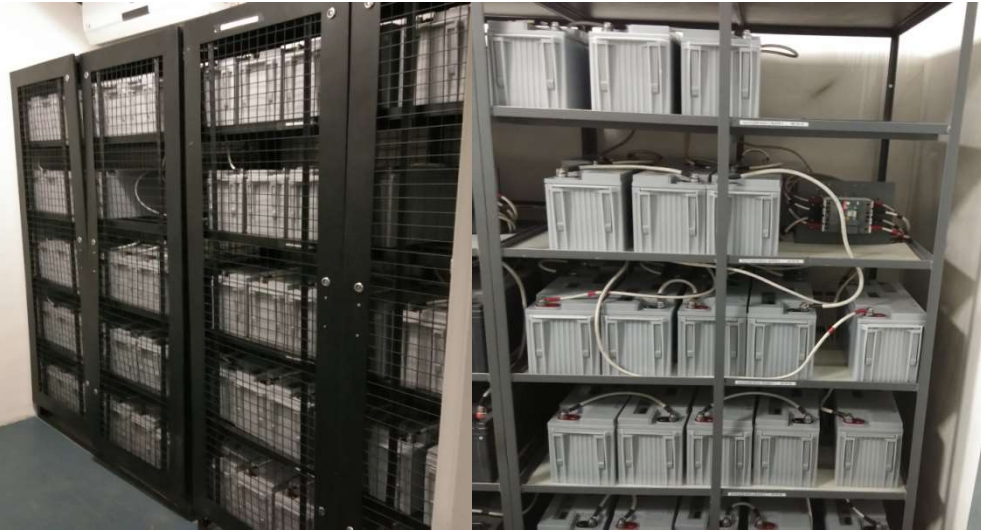
Installed 100AH Battery at Tech Park for Higher Capacity UPS
