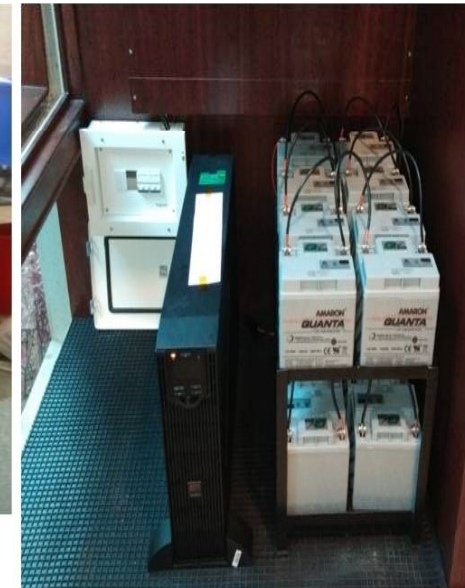
5Kva UPS Installed at Villa
