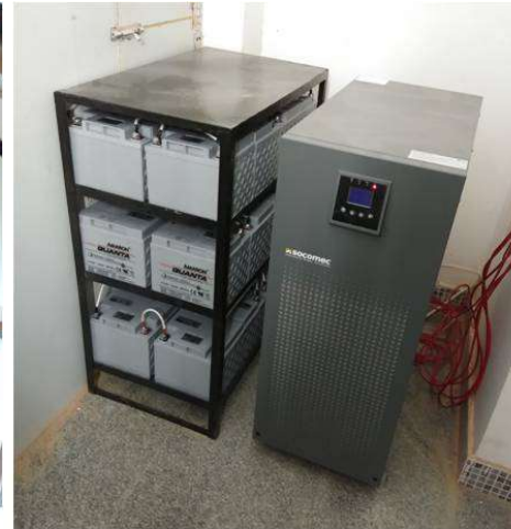
10Kva UPS for Flex Printing Machine
